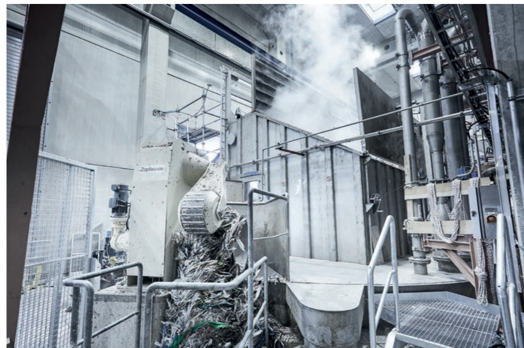
The pulping system with detashing includes a 130 m³ FibreSolve FSR pulper – the largest LC pulper ANDRITZ ever installed in Europe.
