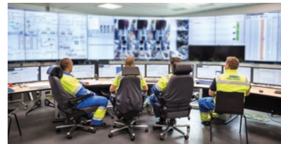
ANDRITZ supplied the Decision Support Wall (DSW) at the woodyard control room, which aids operators and maintenance groups in their daily work. It also acts as a common online remote meeting place for ANDRITZ and the operators.
